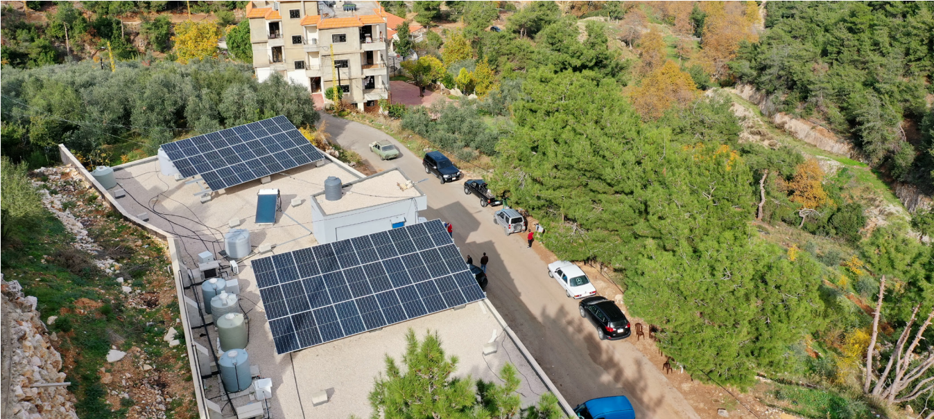
Figure 3. 25-kWp solar PV hybrid on-grid rooftop system, with a 90-kWh battery capacity in Akkar Al-Atika Village in Lebanon, serving the cooperatives building, municipal building and health clinic
