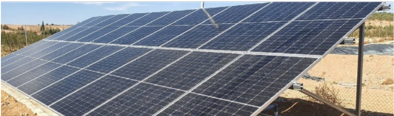
Figure 2. 22-kWp solar PV on-grid ground-mounted system for farm of Saleh Afash Al-Jazi in Al-Achaari Village in Jordan
