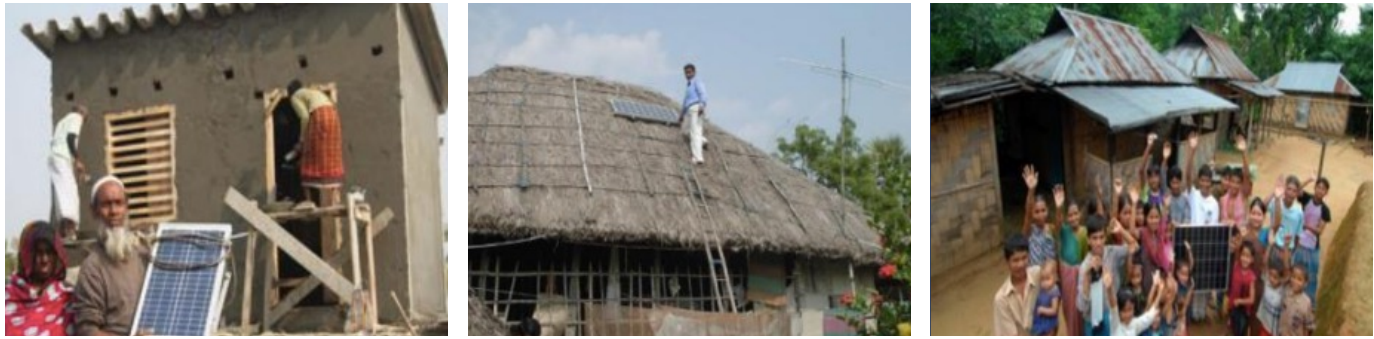
Figure 14. Family installing SHS on their home. Technician installing SHS on a home rooftop. School children excited about a SHS being installed
