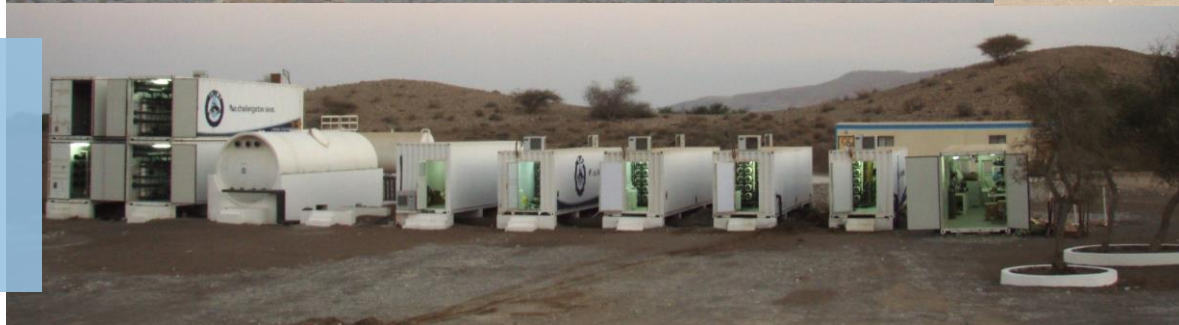
Containerized UP TO 10,000 m3/D
