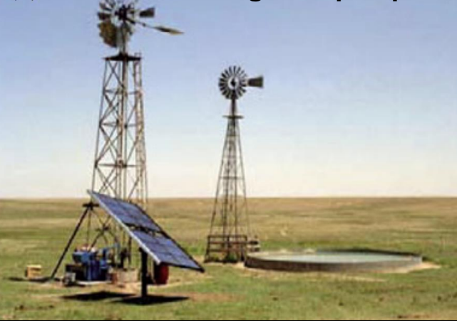
(a) PV windmill integrated pump
