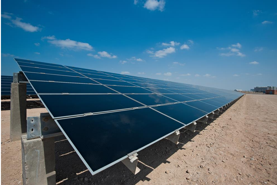
Masdar City: 10 MW PV Operational since April 2009
